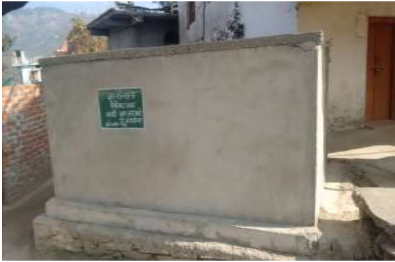
Rain water harvesting tank
